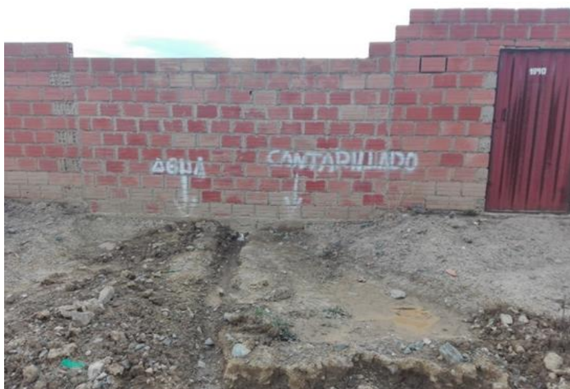
Picture 2: El Alto, Municipal district 7. Nueva Florida housing development. Installation of water and sewerage (Photo: V. H. Perales, 2018)
